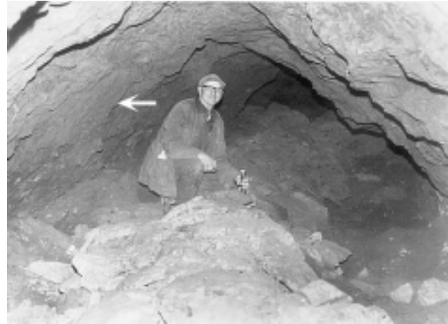
Herman Horstmeyer kneeling on rubble from the collapsed ceiling of the old Coal Butte Mine. The undated photo was likely taken in the 1960s. The arrow points to the approximate position of the ceiling before it collapsed. Mr. Horstmeyer eventually filled in the mine entrances because he was concerned that a child would be killed or injured in the old, unstable workings.
